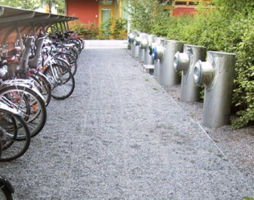
Multiple waste receptacles near the building entry allow for separation of waste by occupants. The waste is conveyed to a central collection point by a suction system.
