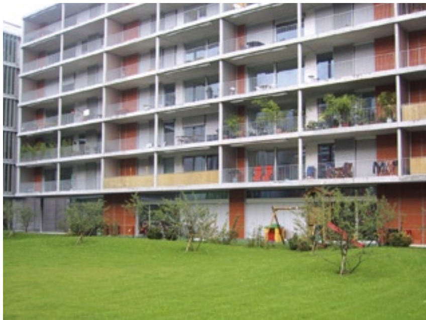
Balustrades in this building are not providing sufficient privacy for some residents.
