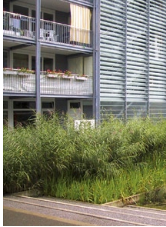
Stormwater from this site is collected and percolates down through stepped levels of reed beds that filter suspended particles and contaminants.
