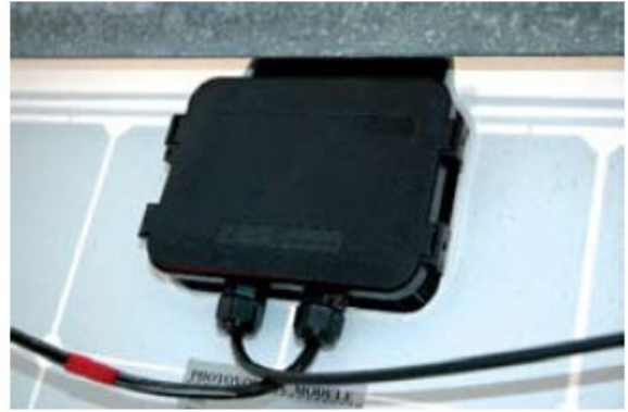
Figure 4: Isolation of PV panels
